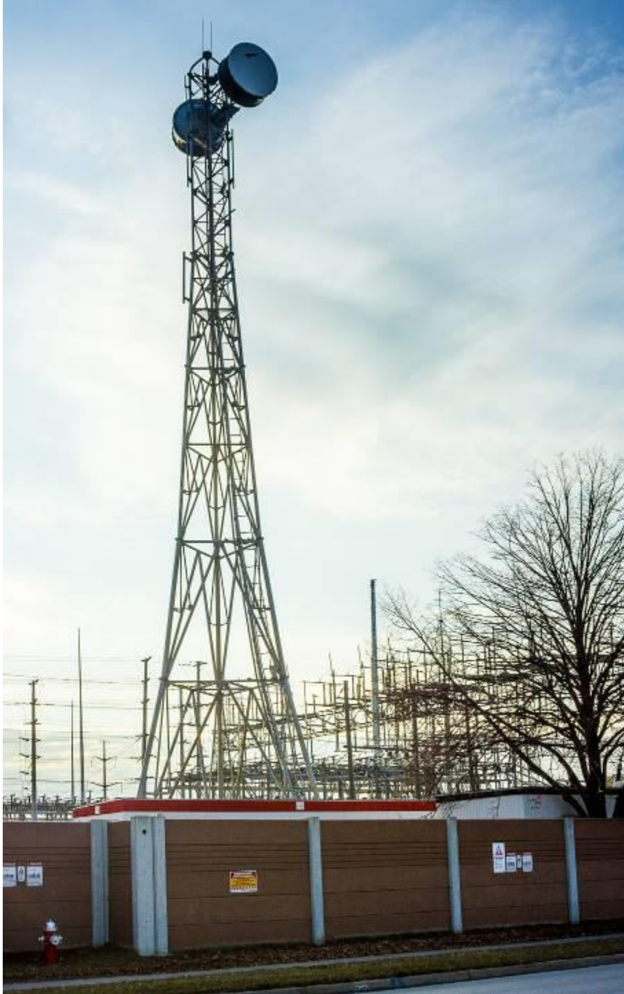
Figure 5: A Typical Telecommunication Tower
